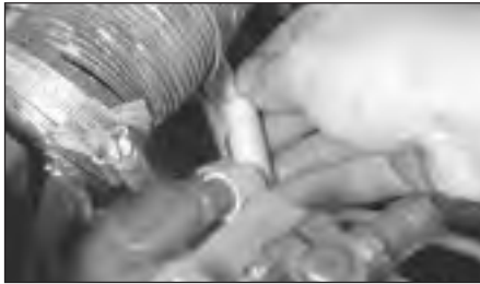
A Check that the HT lead connections at the distributor are clean and secure.
