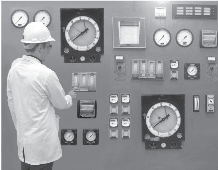
Old analogue control panel
